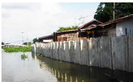
Waterside image after flood barrier.
