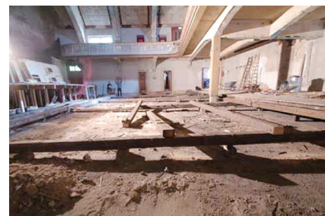
图4 莱比锡灯光剧院更新中的地板 Fig.4 floor under repairing in Leipzig Theater
