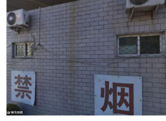
Buildings with unkempt facades
