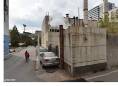
Buildings with damaged facades
