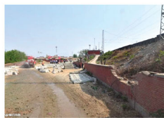
Damaged public interface
